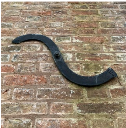
Figure 39: S-shaped iron wall ties are present in many dwellings.
