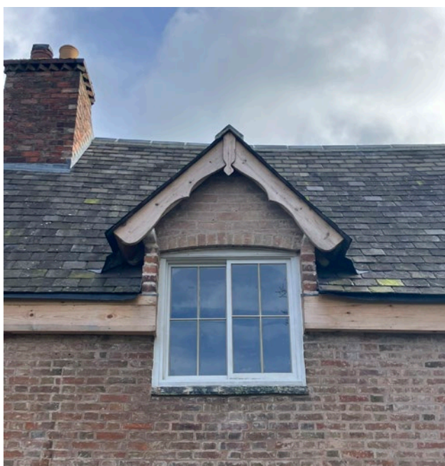
Figure 64: Within Burton Overy, dormer windows are generally small in scale, set down from the main ridge line, with a pitched roof. Any new dormers should reflect this existing character.
